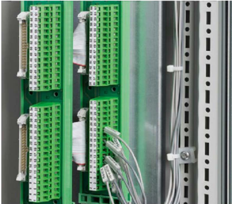
Figura 10-92 Terminal Module Cabinet
