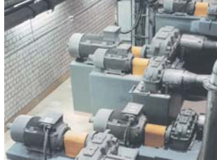
Pumps for water treatment of pools
